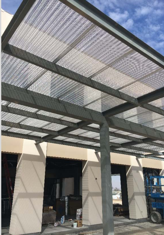
Progress photo of the outdoor dining area trellis for the North County Campus Center cafeteria.
